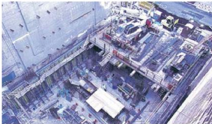
Workers secured the construction site on East 58th Street on Friday, a day after a 'stop-work' order.
